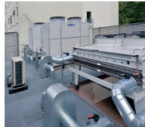
The roof of the transformer building accommodates refrigeration components and supply lines find their place.
