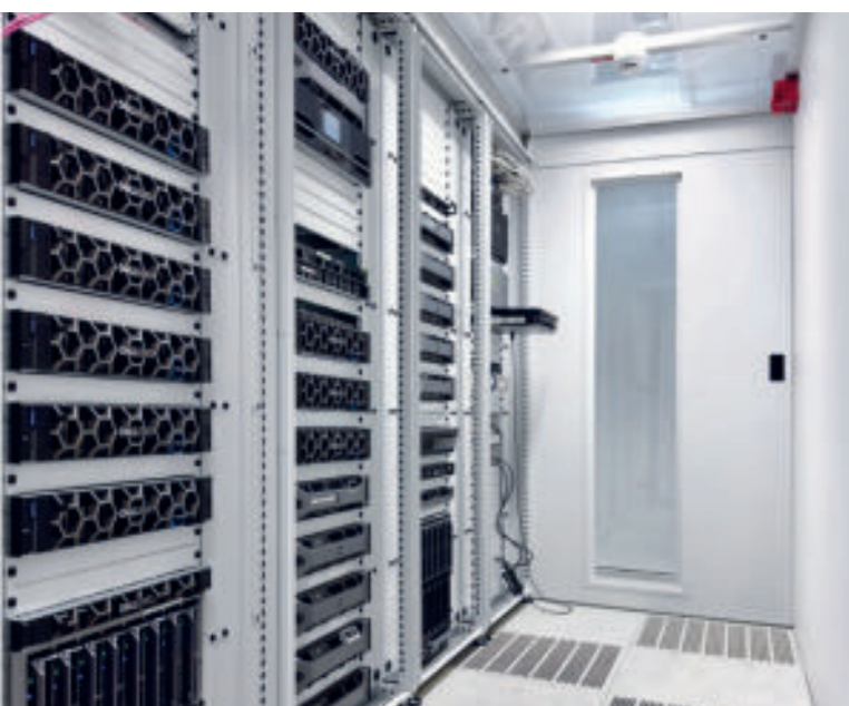
Server racks and server aisle including security door separating the server room from the technical room.
