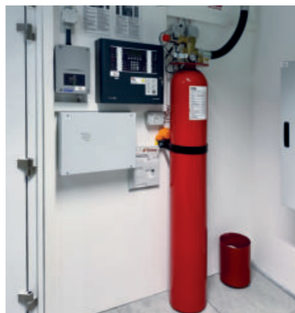
Early fire detection system including NOVEC 1230 fire extinguishing system with fire alarm system.
