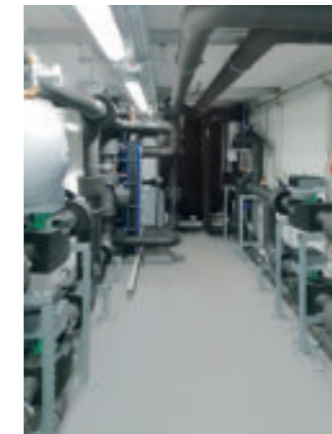
Refrigeration center of the data center on the Mezzanine floor.
