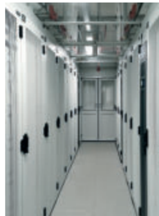
Strict separation of hot and cold air through cold aisle containment.
