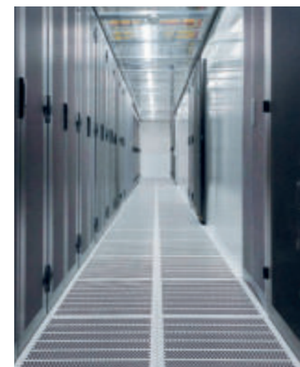
Cold aisle containment of the o2 Telefónica test lab data center in Munich.
