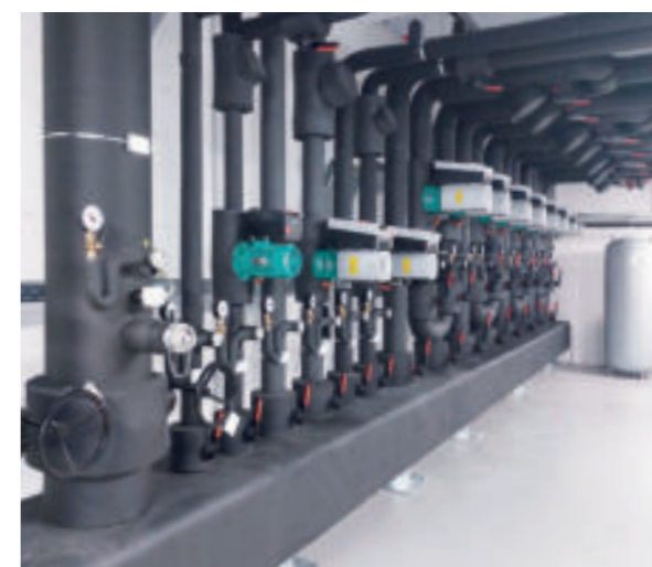
The refrigeration system ensures adequate cooling of the IT infrastructure.
