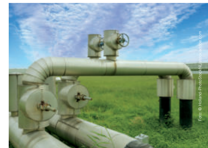
The waste heat can, for example, be fed into a heat network for the municipal heat supply.
