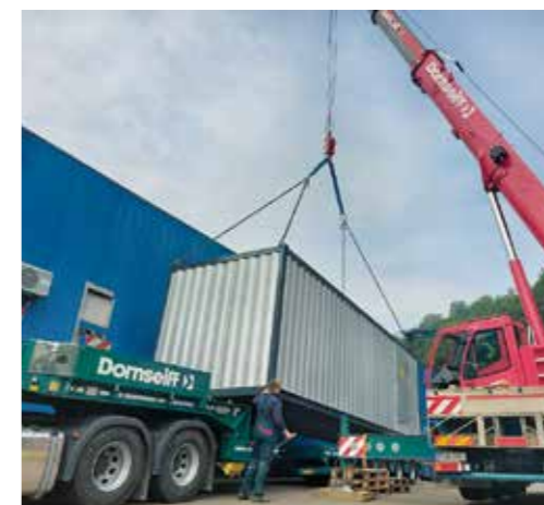
The data center container can be transported by trucks.
