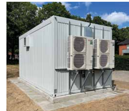
Alternate data center in a container.
