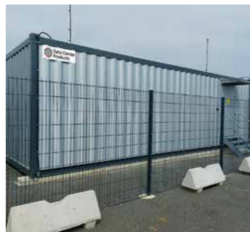
The container data center offers maximum availability and secure protection for sensitive production data.
