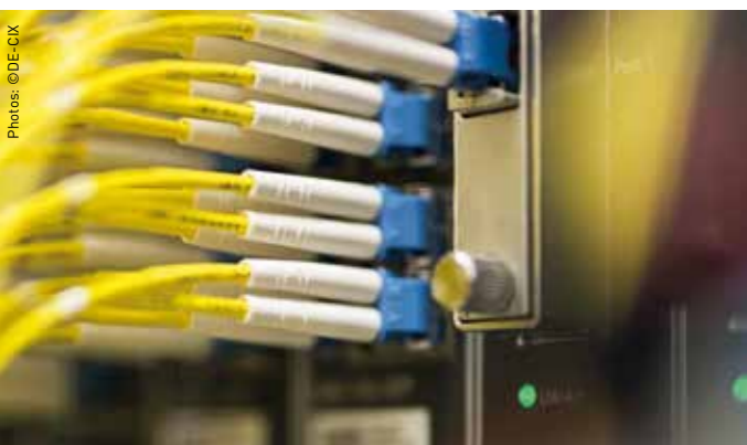
At the Internet nodes, DE-CIX cables and patch panels are used to interconnect various networks.
