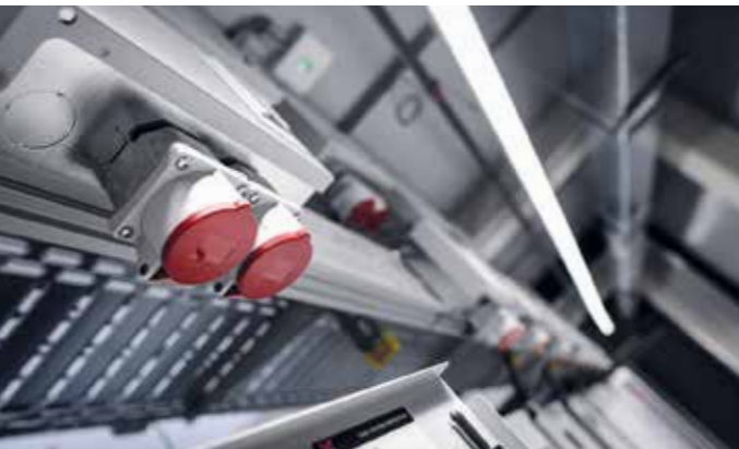
All the trades interlock perfectly: state-of-the-art technology and a special sustainability concept ensure secure data center operation.
