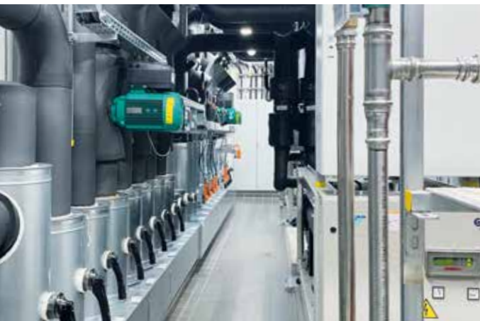
Thanks to targeted reengineering measures, RZservices was able to achieve significant energy savings in the Hörmann data center.
